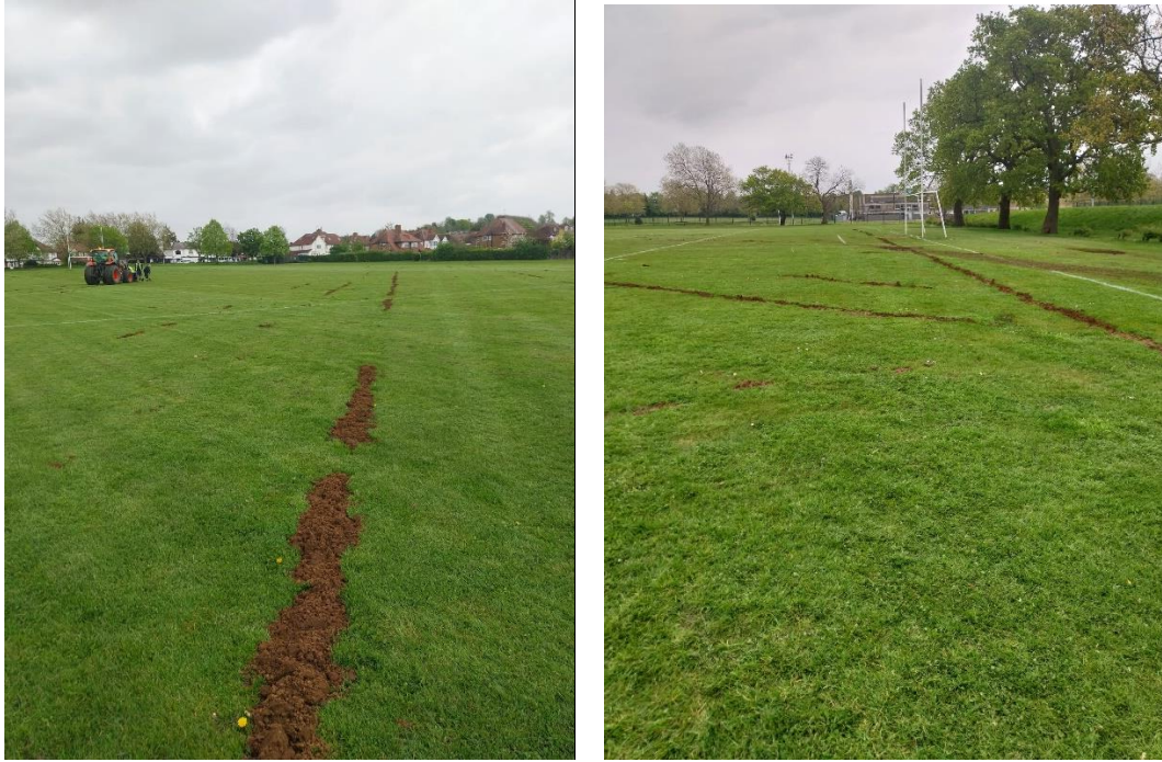
Figure 16 Image of Vale Farm Gaelic Pitch - Drain lines being filled with top soil
